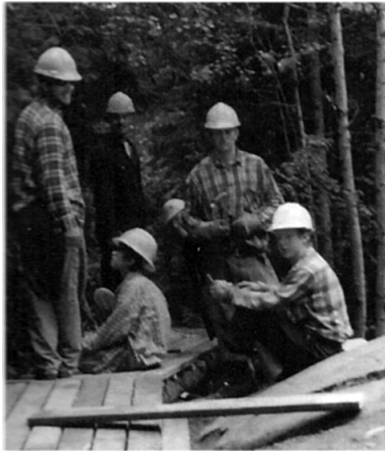
Damon McCreary, Roy Freda, and Bill Byl repair the boardwalk with staff John Barbon and Bill Mantha.
